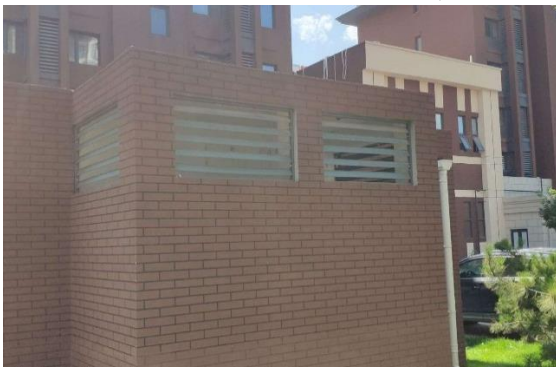
地块排风竖井
